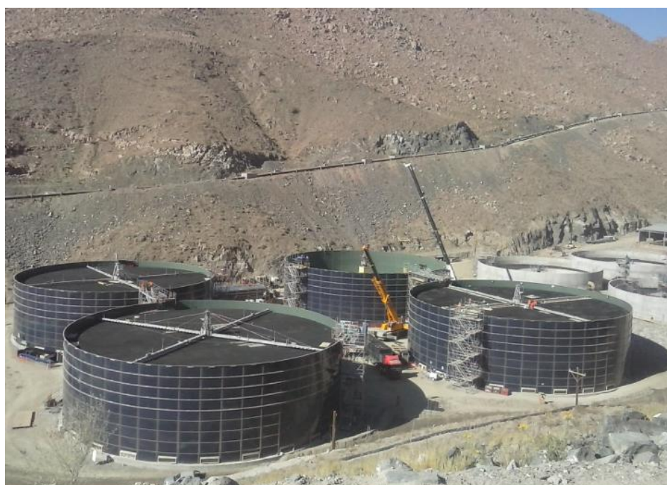
Figura N°01: tanques percoladores o trickling filter.
