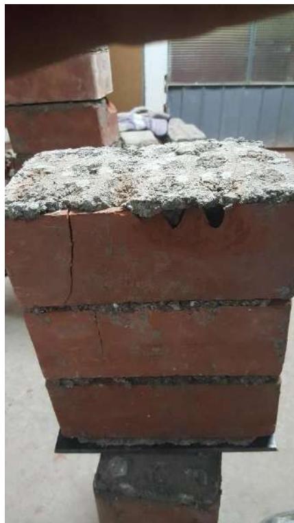
Presenta falla vertical
