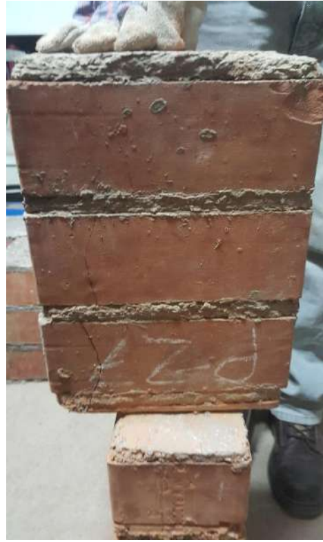
Presenta falla vertical
