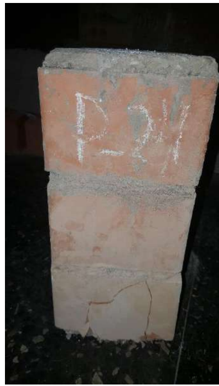
Presenta falla vertical
