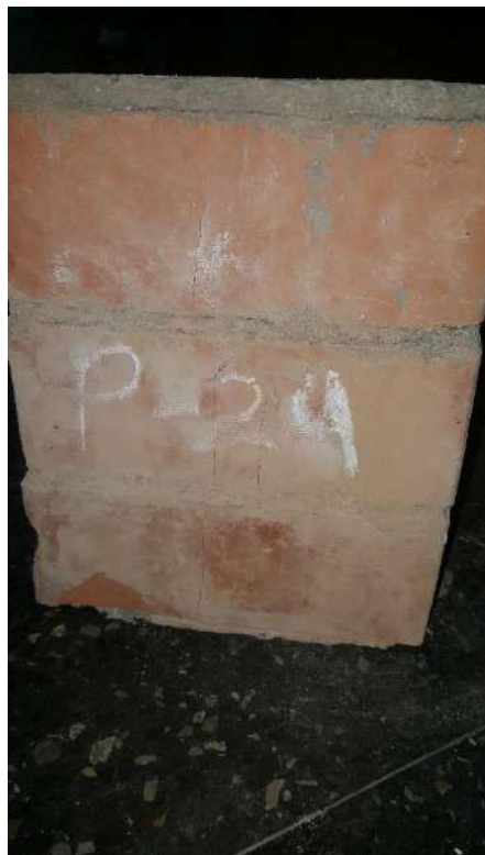
Presenta falla vertical
